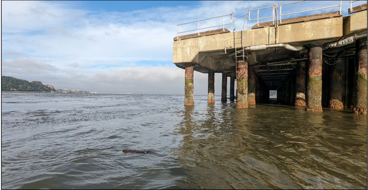
Photo 7. Looking westward along the existing main pier where the TSGB would normally be docked. This pier will be demolished with a new, larger pier constructed on the outboard side (left).
