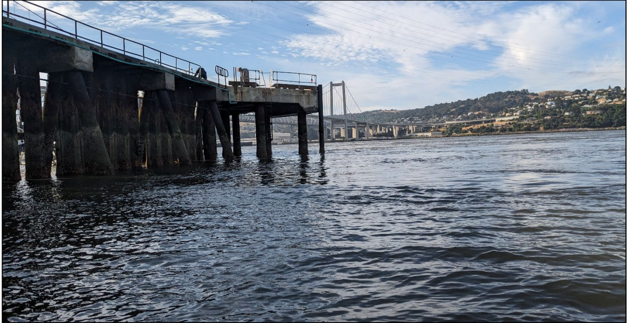
Photo 1: Main pier structure used for docking of the TSGB. Looking to the east toward the Carquinez Strait.
