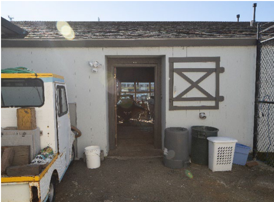
Figure 8: South end of the east façade of the transverse wing of the Boathouse, looking west.
