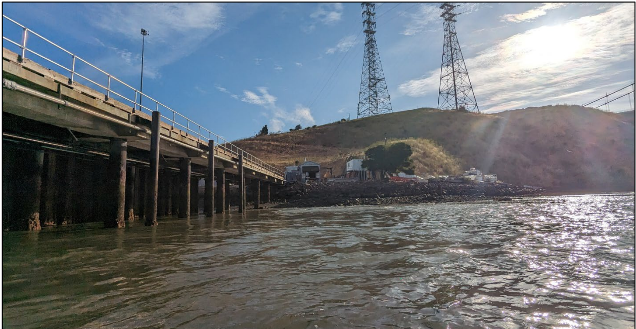
Photo 2: Existing trestle as it approaches the shoreline. Trestle to remain in place.
