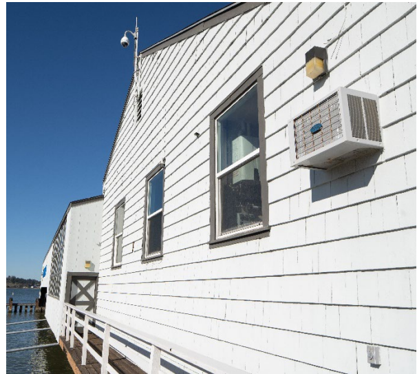
Figure 13: West façade of sail loft portion of the Boathouse. Looking slightly northeast.
