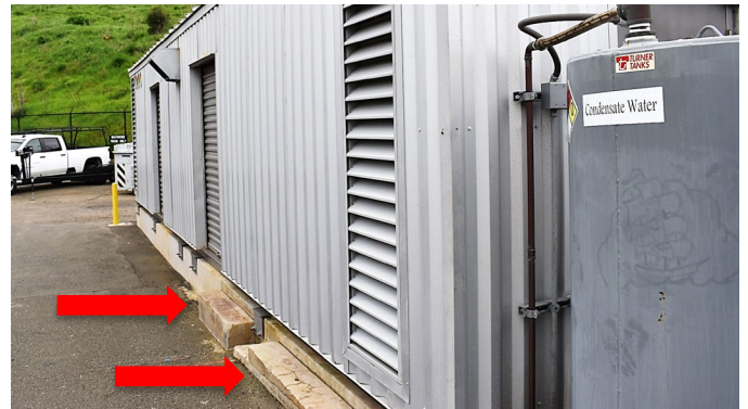
Figure 9: Oblique view from the southwest corner of the building, view northeast. Arrows indicate concrete steps.
