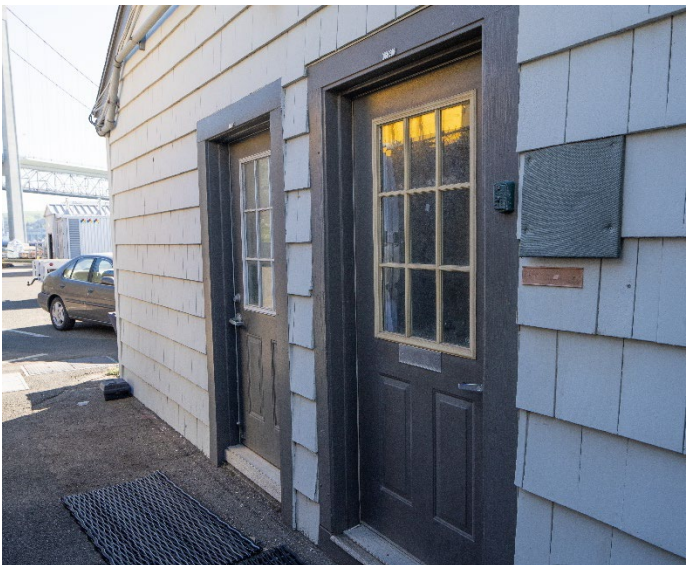
Figure 6: Detail of doors at east façade of the sail loft portion of Boathouse, looking south.
