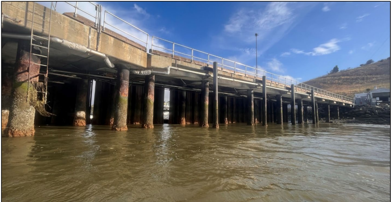
Photo 4. Closer detail of piles under the trestle including sheetpiles which form the breakwater to protect the current boat basin.
