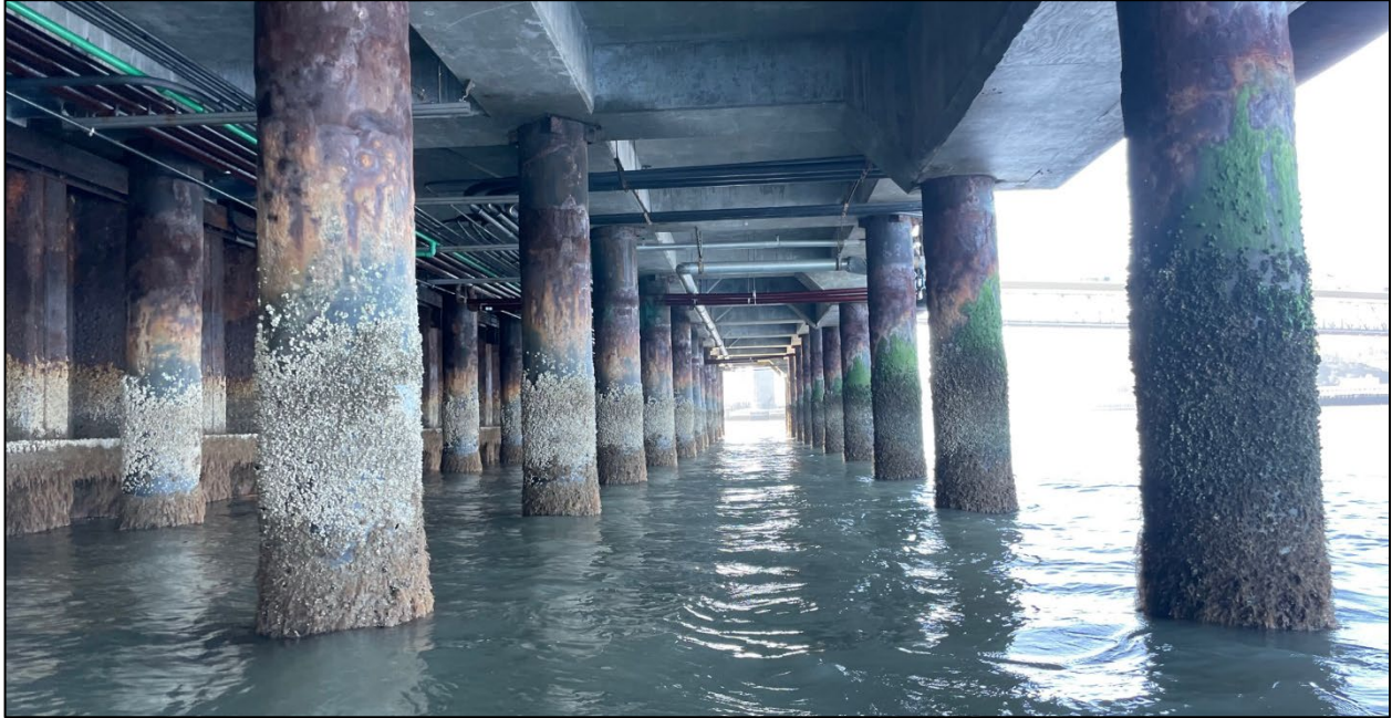
Photo 5. Beneath the main pier. The deck above is solid concrete to allow for heavy equipment and vehicles to load and unload cargo from the TSGB. A similar deck will be necessary for the new pier under the Proposed Project.
